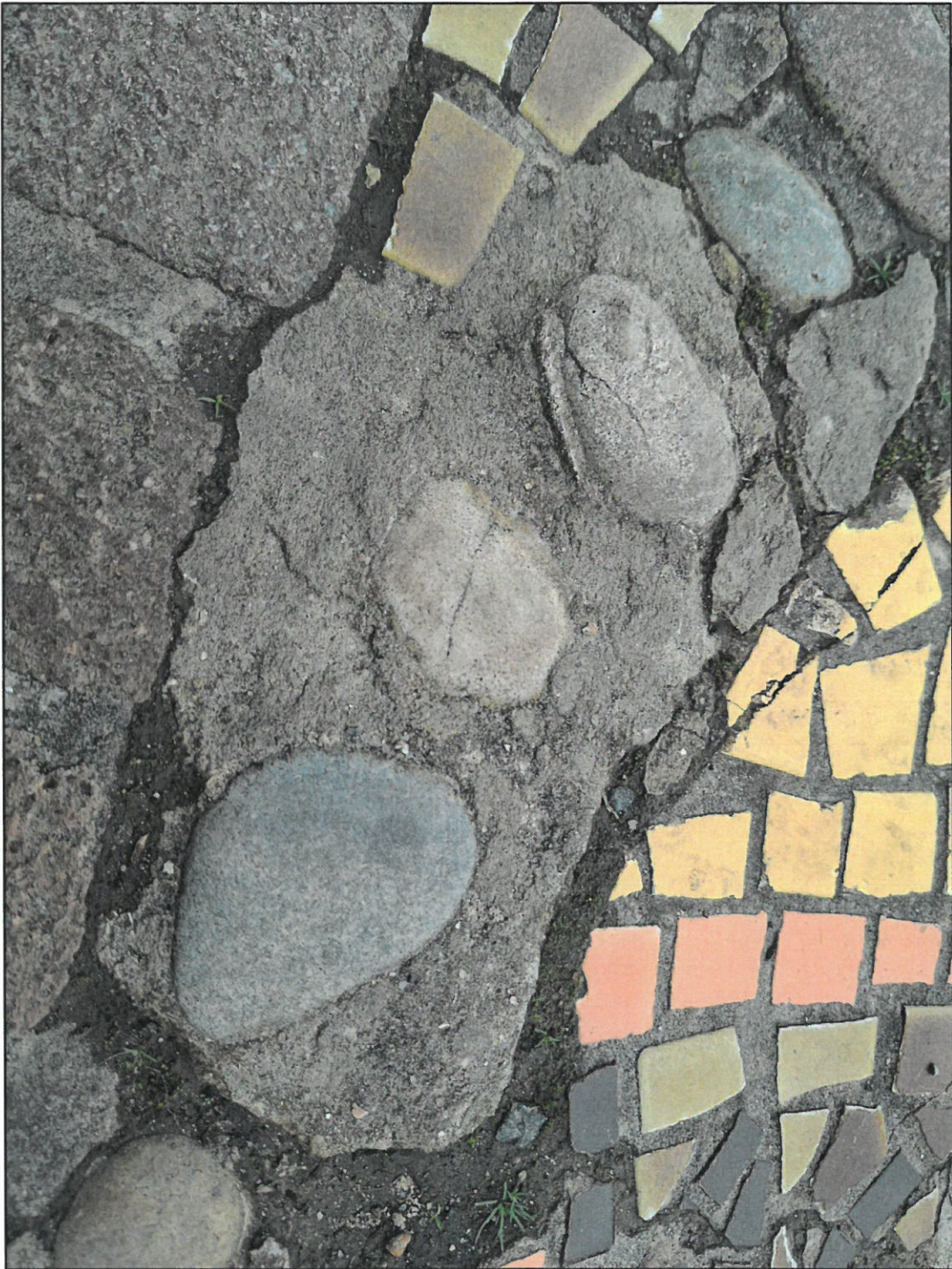
Some cement repairs have been done to a poor standard
