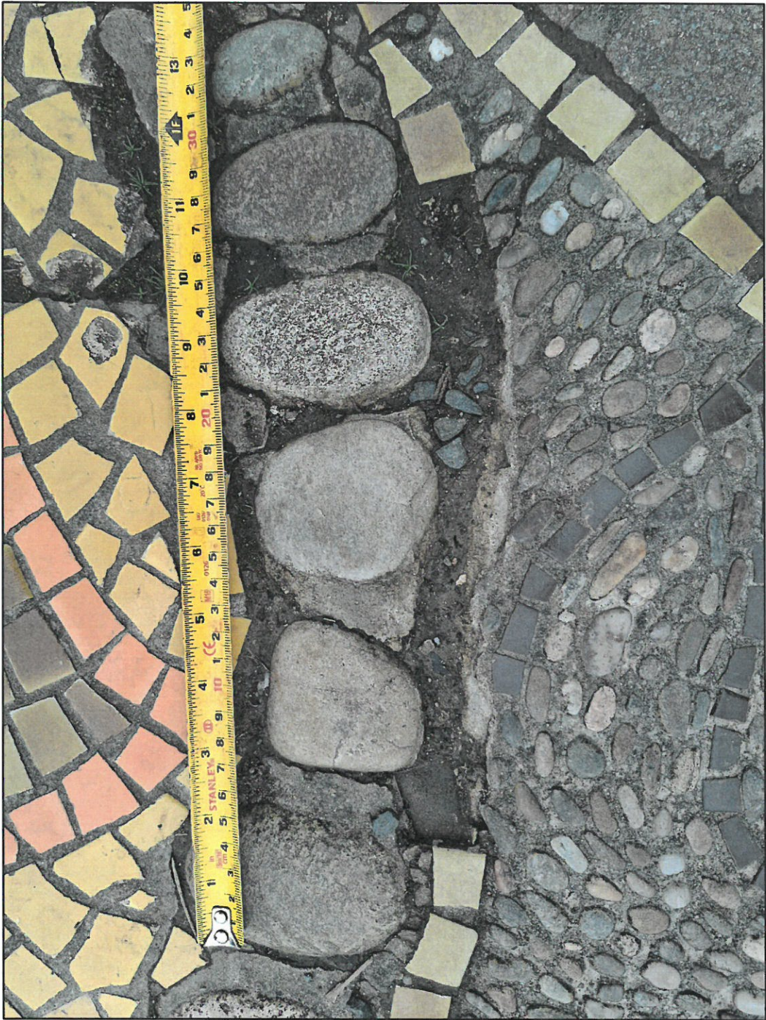
Numerous glazed ceramic tesserae are missing
